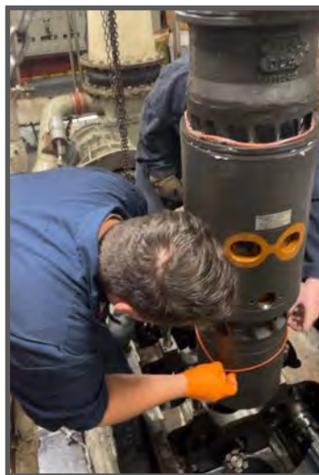
Cylinder liners absorb much of the friction from the inner workings of the diesel engine and are designed to be swapped out when worn. Installing new cylinder liners is a big job. Here, MARMC Sailors ensure that the O-rings are installed properly, so crank case oil doesn't leak. (Photo by EN1 (SW) Kevin Mellor.)
