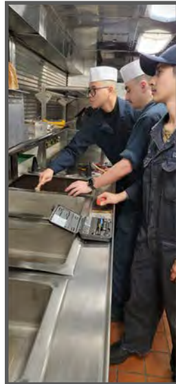
Right: EM3 Julian Aranda, EMFN Nam Trung Pham and FN Jace Peterson listening to instructions on how to install a new steam table.
