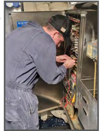
EM3 Kaleb Stryd from USS New Orleans (LPD 18) taking readings on relays for the Gaylord Vent System Washdown. (Photo by Rizalito Antonio.)
