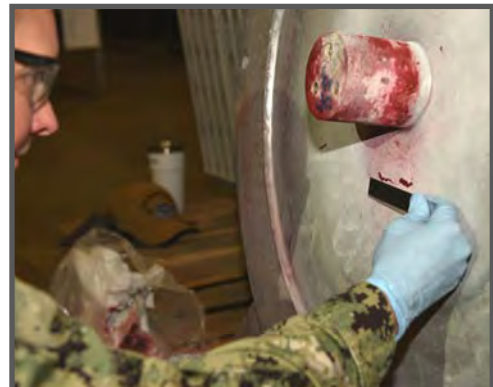
Below: Hull Technician 1st Class Petty Officer Jennifer Schleuning measures cracks that are normally invisible to the naked eye on an upper platform for a ship's brow while conducting non-destructive testing. Schleuning was selected as OPNAV Shore Sailor of the Year for 2023. (Photos by Scott Curtis, SERMC PAO.)
