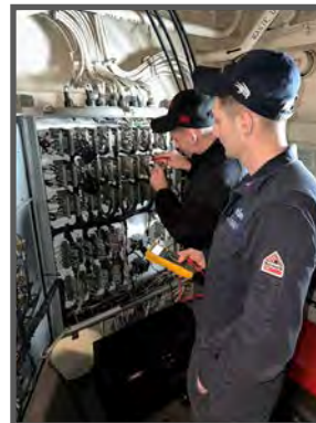
EM2 Dmytro Tsyganovskyi and EM3 Kaleb Stryd are taking readings and checking connections for the solenoids on the ship's stern gate. (Photo by Rizalito Antonio.)
