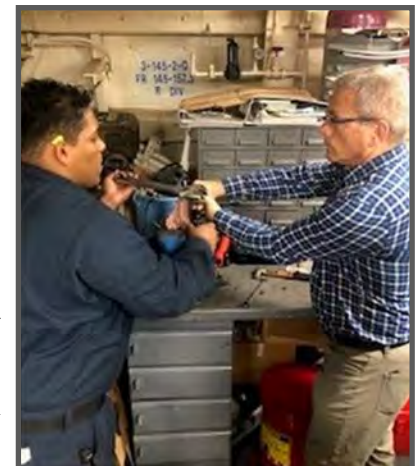
EN2 (SW) Antonio Ayala from Los Angeles, Calif. attempts to back out the yoke bushing nut on valve 2B-PFS-V-30B as NAMTS Afloat Outside Machine mentor Mike Dengage holds the valve stem. 2B-PFS-V-30B is frozen in the open position. (Photo taken by Rick Smith).
