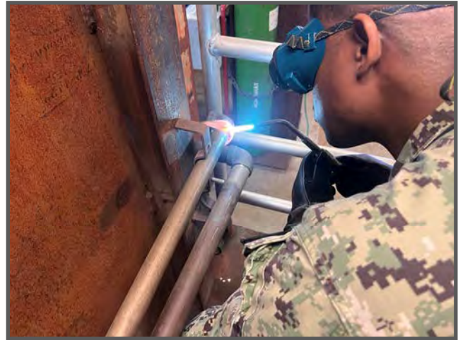
DC2(SWHT2(SW) Lorey Slater conducting an oxyacetylene brazing of an insert-type pipe socket as he works through the NAMTS General Shipboard Welder/Brazer JQR. (Photo by HT1(SW) Malcolm Luckie.)
