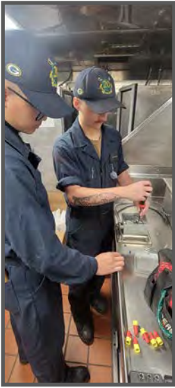
Left: EMFN Nam Trung Pham and FN Jace Peterson Making final connections on a new steam table.
