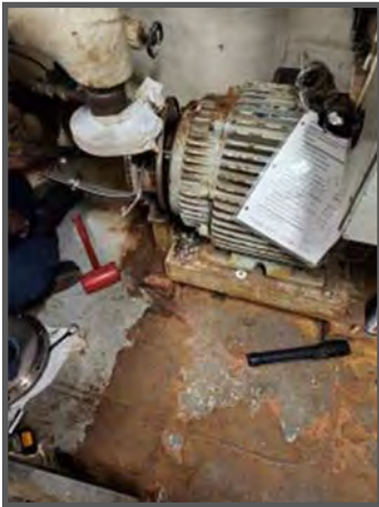
MM2 Armstrong Calixte from Port Au Prince, Haiti removes the suction cover for Nr. 5 Chill Water Pump.
