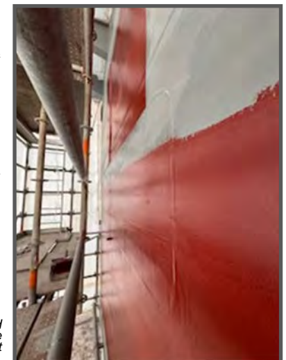
Patches were sealed and primed. Ship's force will apply the topcoat to match the area.
