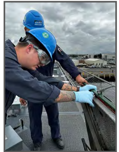
DCFN Noah Steadman (front) and DC3 Devin Rivers conduct an inspection of the gasket on a Quick acting water tight hatch on board an Independence variant LCS.
