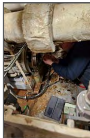
MR2 Michael Schomisch from Cleveland, Ohio taking inside dimensions of No.4 Chill water pump casing wearing rings for fitment and machining of impeller wearing rings.
