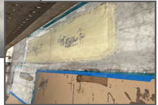
Below: This patch was a combined length of 12.25 foot long patch, mean while the three patches below are temporarily covered for protection.
