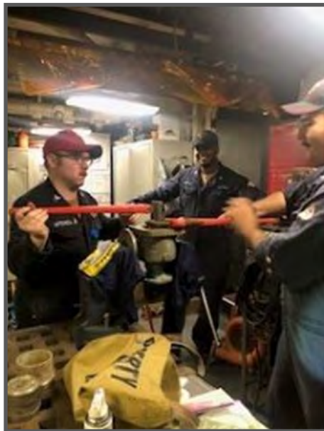
HT1 Nash Mitchell from Spokane, Washington and HT2 Roman Fuentes from Houston, Texas remove the seat from relief valve FL-V-2-102-13, Nr.2 Flushing water station.
