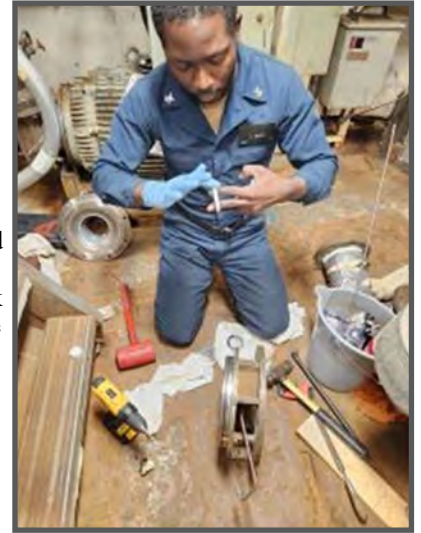
MM2 Armstrong Calixte from Port Au Prince, Haiti lubricates the mechanical seal cartridge prior installation on Nr.4 Chill Water Pump.
